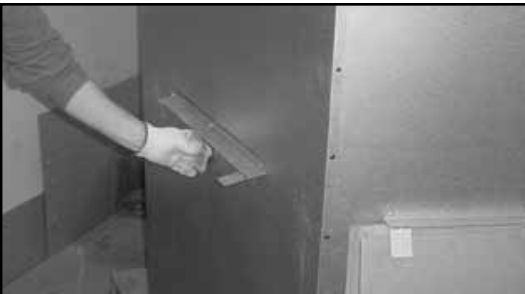
Figure 7.2 Bend Refractory Brackets Back Down
