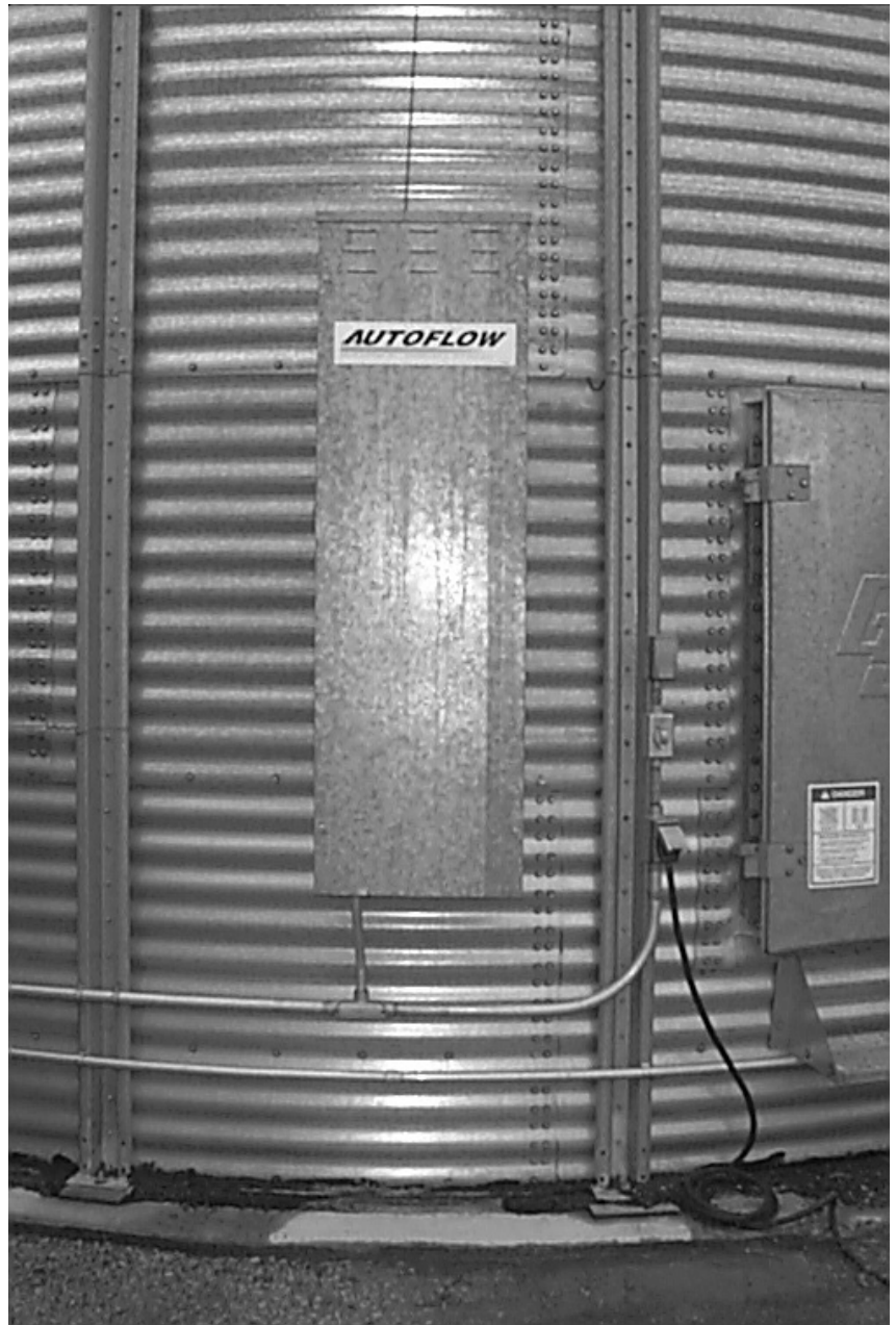
Actuator Control Box Mounted to Bin
