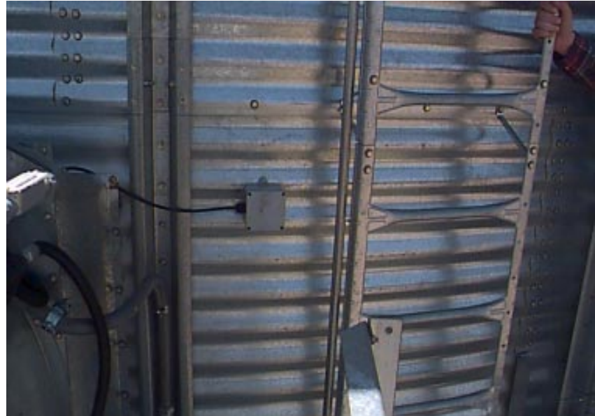
Plenum temperature sensor on the bin sidewall.
