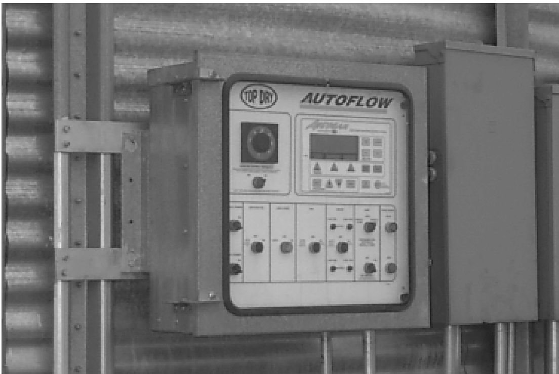
Autoflow Control box mounted on bin.
