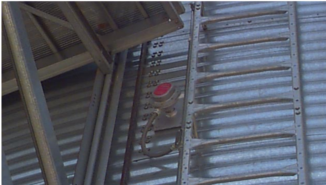
Storage chamber rotary switch.
