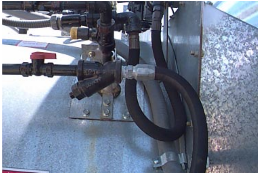
LP line field connection.
