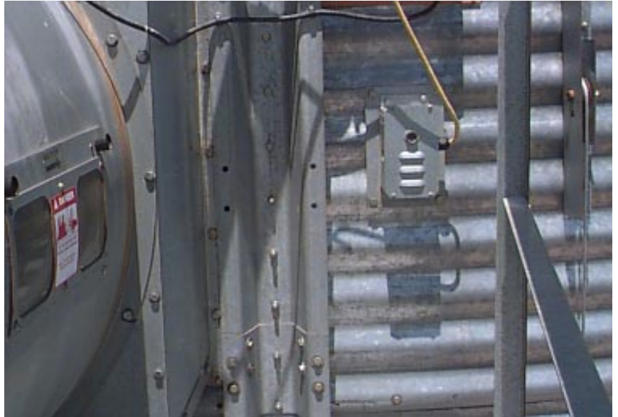
Airswitch mounted on the bin sidewall.
