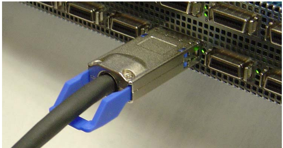
Figure 1-11: Fully Installed IB Cable with Pull Connector
