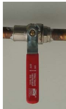
Photo 2b: Ball valve: closed position
